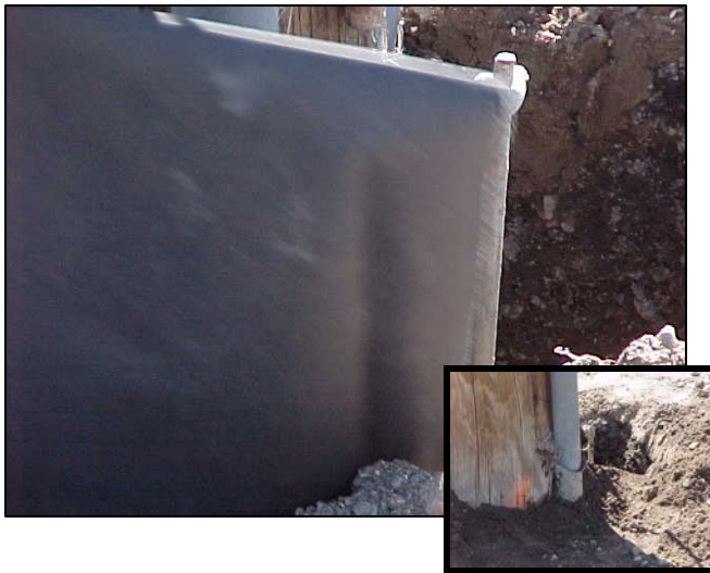
Photo 3. A wrapping or bandage is place over the treated area and stapled to the pole. The bandage usually consists of a plastic film and a backing of stiffening paper. The film acts as a moisture barrier between the soil and treated pole. The excavated area is backfilled and a date tag is affixed to the pole
