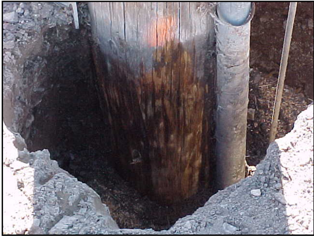
Photo 1. Soil around ground line is excavated to a depth of 18 inches and all loose dirt is removed from the pole with a wire brush.
