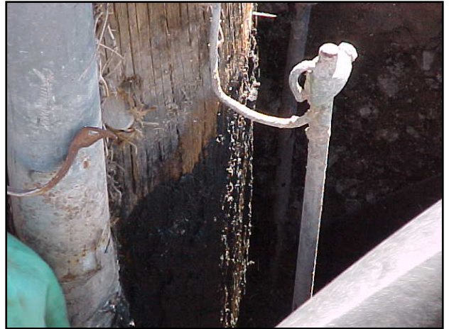
Photo 2. An external preservative is applied to the ground line area of the pole with a long-handled brush. The preservative is liberally spread into the checks and cracks to a thickness of 1/16 inch
